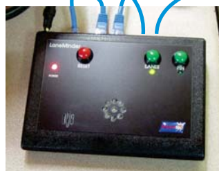
Control Module at Front Desk
